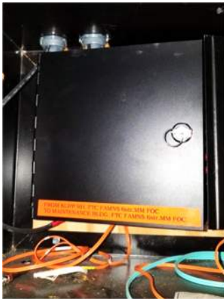
Figure 26: Data termination cabinet.
