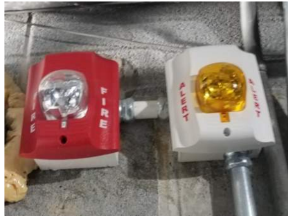
Figure 27: Fire alarm and mass notification devices.
