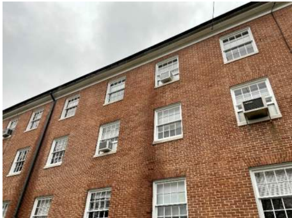
Figure 3: West wall upper showing wet areas from gutter and downspout leaks.
