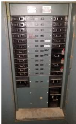
Figure 17: Main distribution panelboard.
