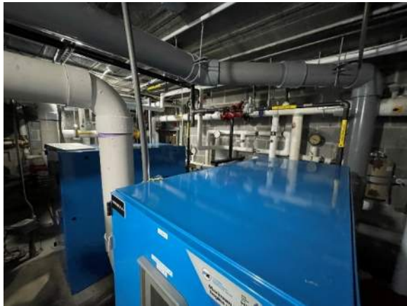
Figure 15: Basement boiler room.
