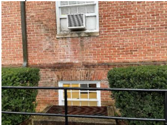
Figure 5: North wall and window water damage.
