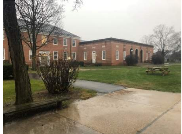
Figure 2: Water ponding, large gaps in pavement in front of Foxwell-Moylan Hall (looking SE toward the Ely building).
