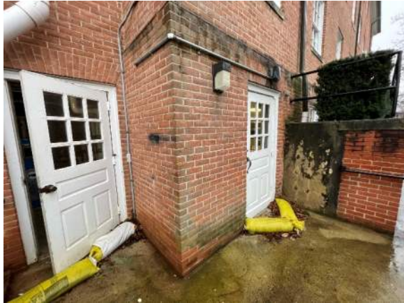
Figure 1: Basement areaway at northeast corner, note doors are sandbagged.
