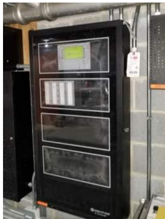
Figure 28: Fire alarm and mass notification panel.
