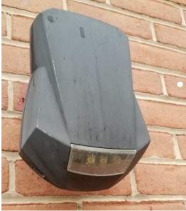
Figure 24: Typical exterior wall lighting.
