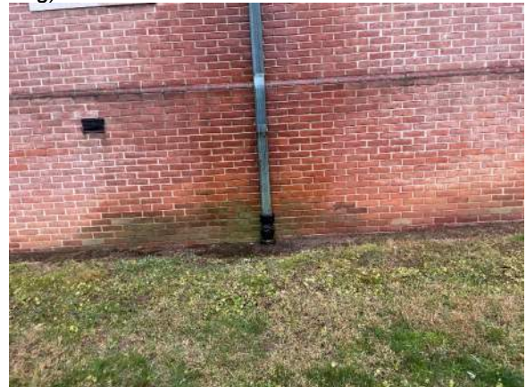
Figure 4: West wall upper showing water staining and erosion at wall base.
