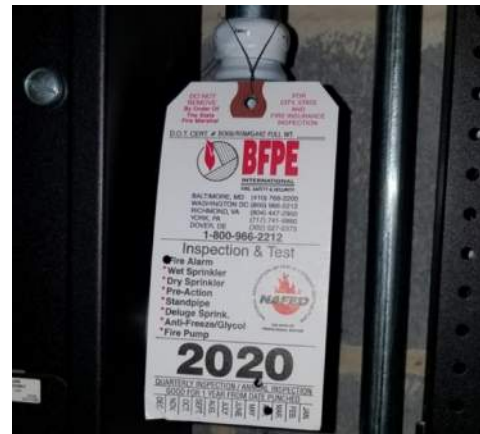
Figure 29: Fire alarm inspection tag.
