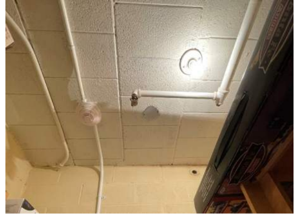
Figure 14: Underside of Celldex structural planks which is the finished ceiling in most spaces.
