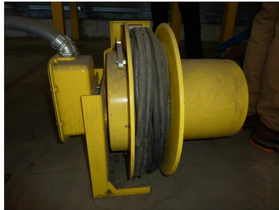
TYPICAL CABLE REEL MHRF & LRT RAIL FACILITY
